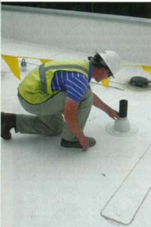
■ Joe Baker of ADC Engineering checks for roof damage during an inspection. Photo courtesy of ADC Engineering.
