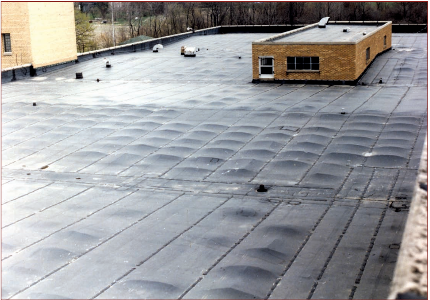
Dimensionally unstable foamed plastic insulation resulted in a failure investigation at this plant in Michigan. (Photo courtesy of Roof Engineering Inc.)
