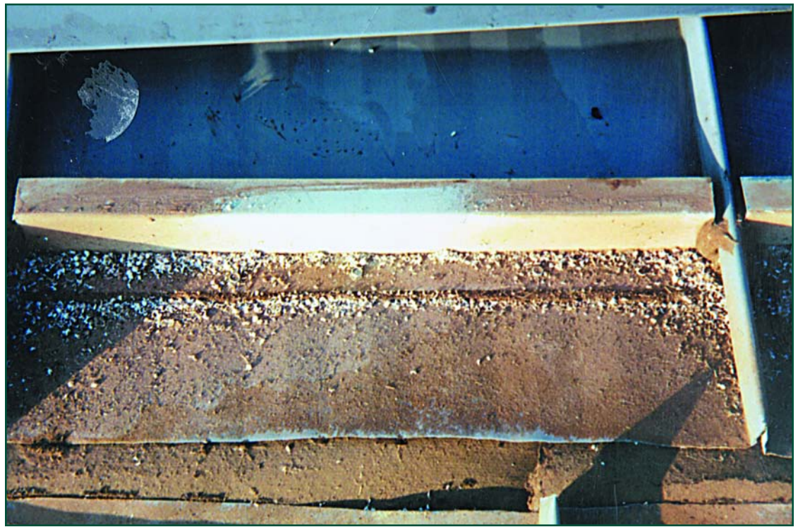
Figure 2 — Close-up view of the metal roofing panel and closure and ridge cap flashing. Water and debris stains are clearly visible. Areas showing debris are supposed to be watertight.
