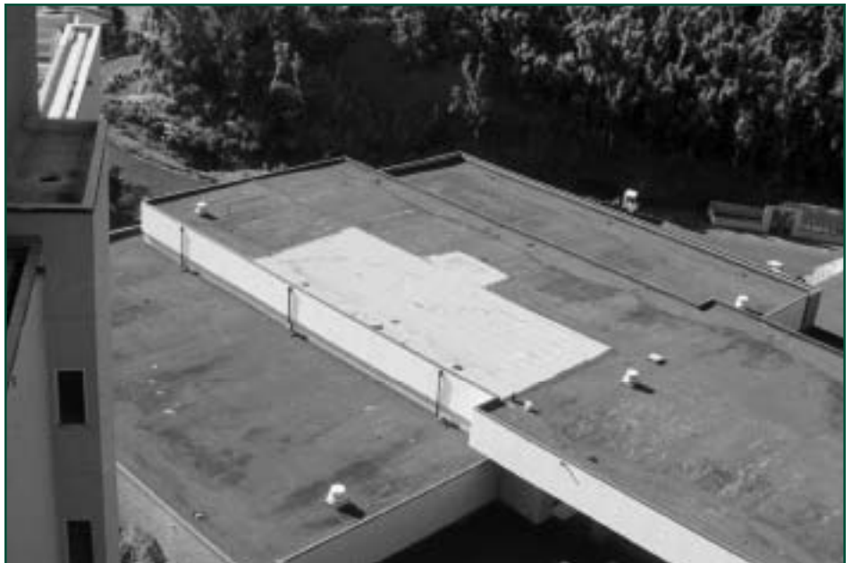
Figure 4: Damage initiated near two roof drains with adjacent through-wall overflow scuppers midway along the windward side of the building.
