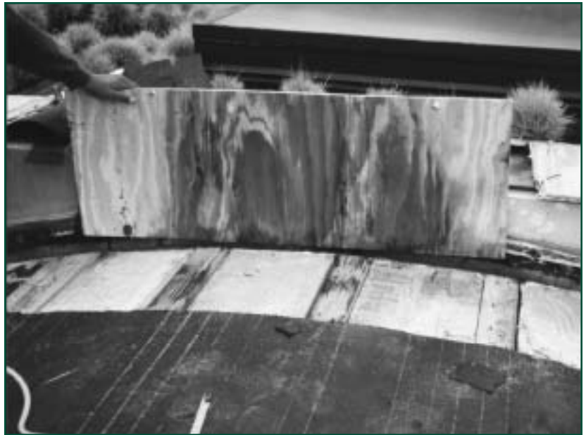
Figure 8: Saturated plywood conditions uncovered near tops of barrels.
