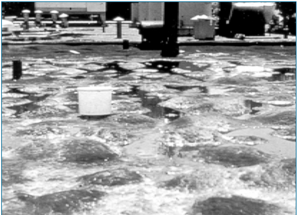
Loosely scripted RFPs, lacking a well-defined scope, can result in an installation or service of questionable integrity. Building owners and their representatives need to be specific when soliciting service providers of any discipline.
