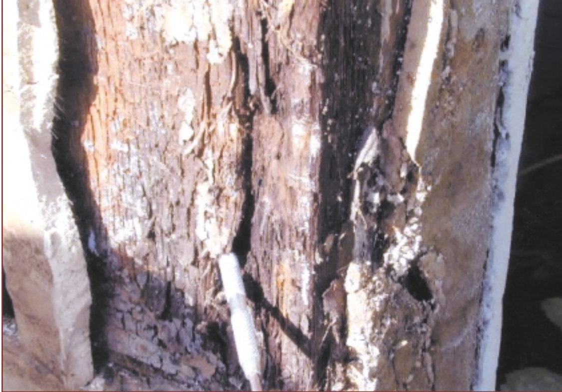
Figure 2: Severe deterioration at unvented “cold wall” clad with stucco on both sides.
