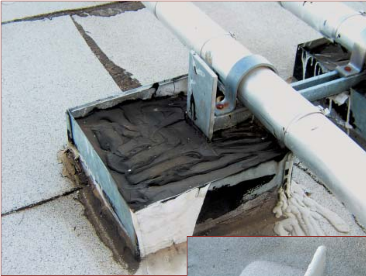
Old pitch pan with dried asphalt mastic.
