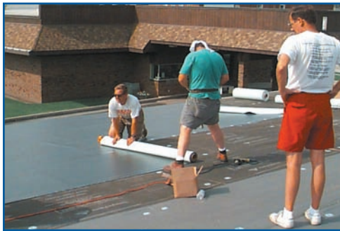
Peter Garrigus of Trufast (formerly of Stevens Roofing) and Dave Scott roll out TPO sheets.
