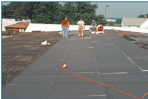
Layout of "cool black" TPO sheets on west side of church roof.
