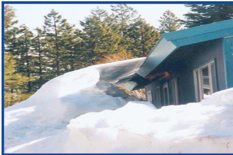
Photo 2: Dormers can be torn off.
