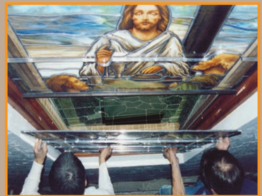
Each panel is secured separately. Small ventilation screens or "breathers" have been inserted into the frame to release heat and moisture from between the existing and new glazings.
