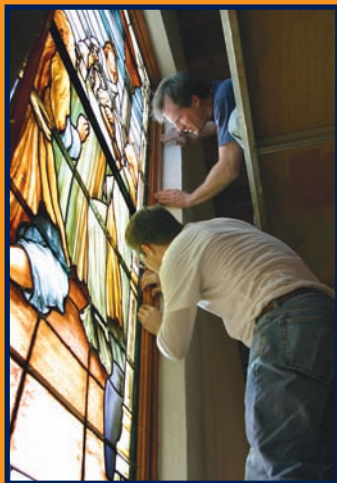
Finish trim is reinstalled after the window is in. The dark bar in the center is the T-bar, which was added.
