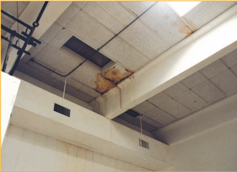
Apparent ceiling leak. (Photo courtesy Fincastle Engineering.)
