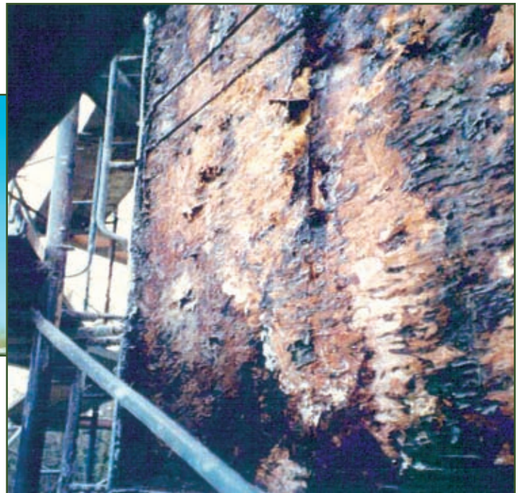
Exterior sheathing damage from excess moisture in wall assembly.
