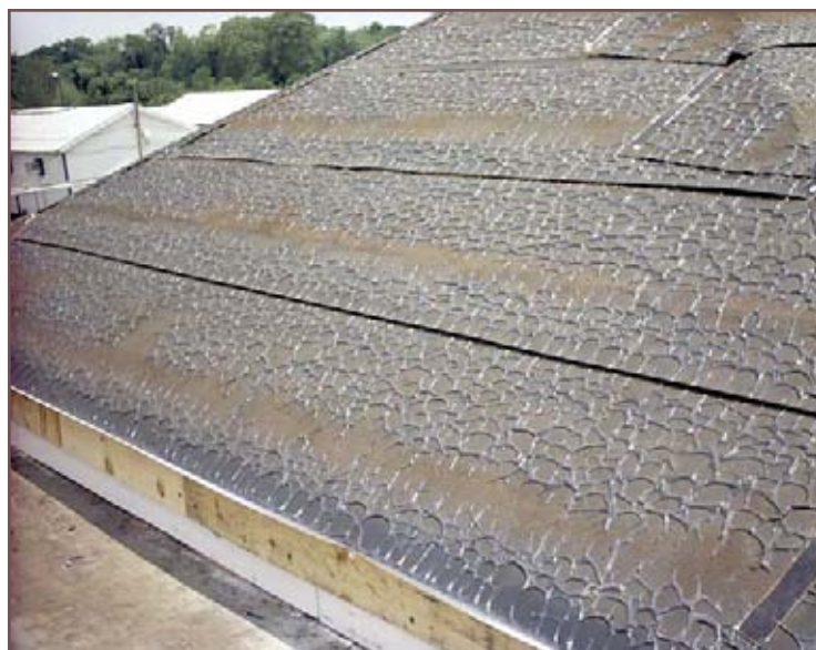
Wrinkled rubberized underlayment due to overexposure.
