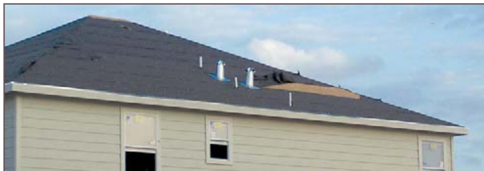
Felt underlayment displaced by wind.
