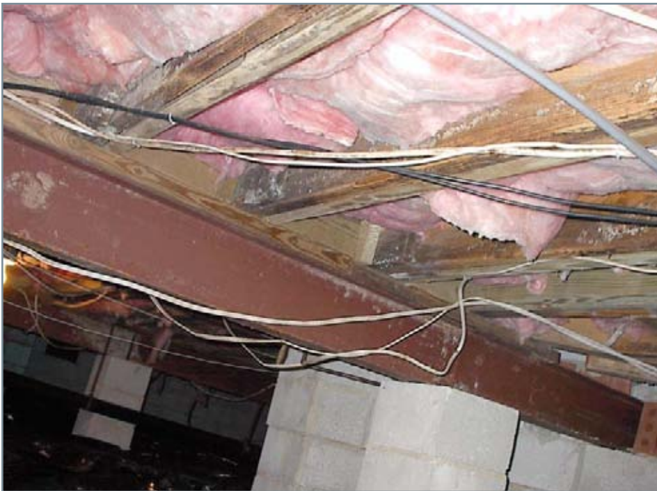
Mold and soft rot on floor joists in crawl space.
