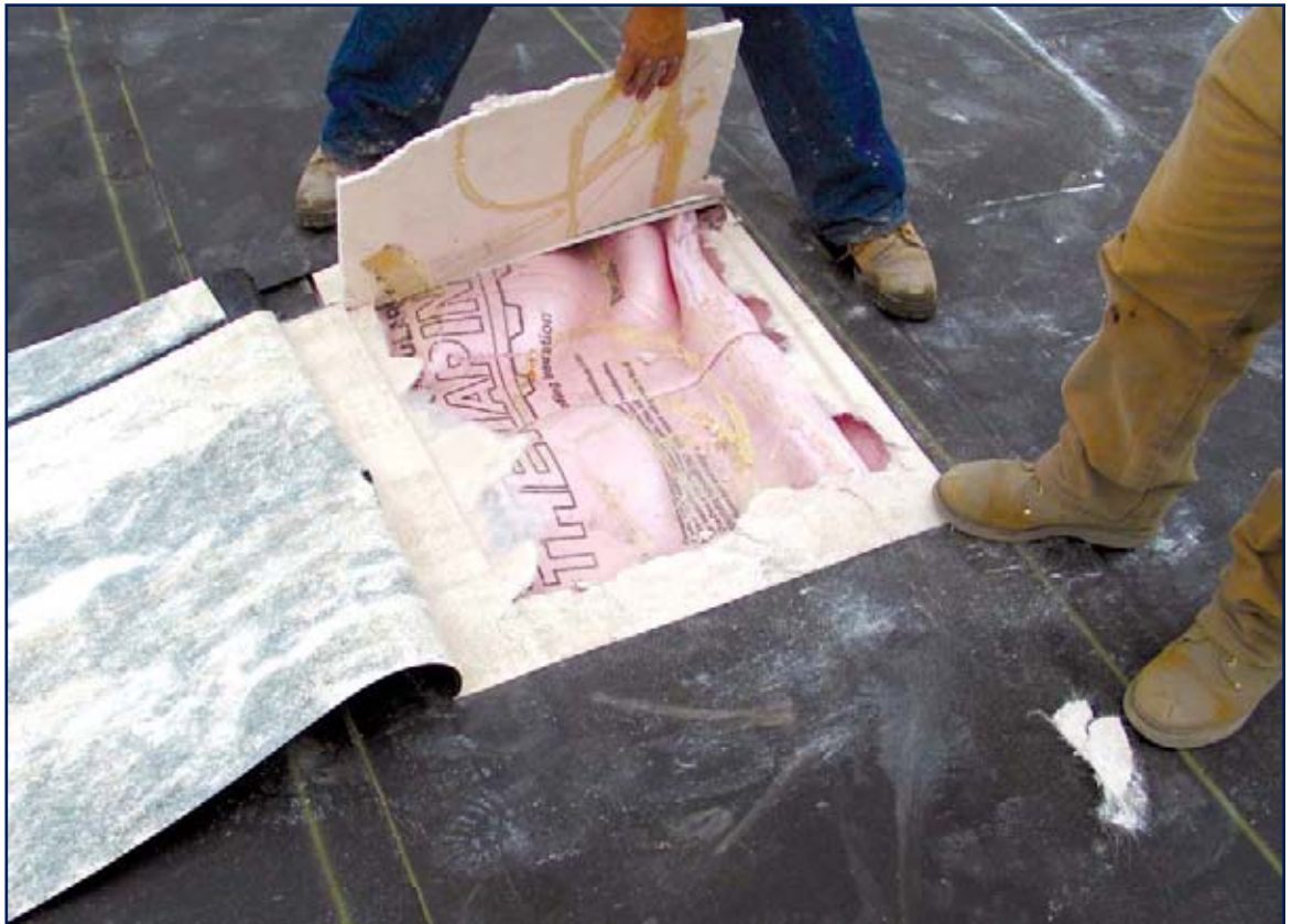
Wrinkling and curling in the EXPS-tapered roof insulation below the 1/2-inch, glass-faced gypsum coverboard.
