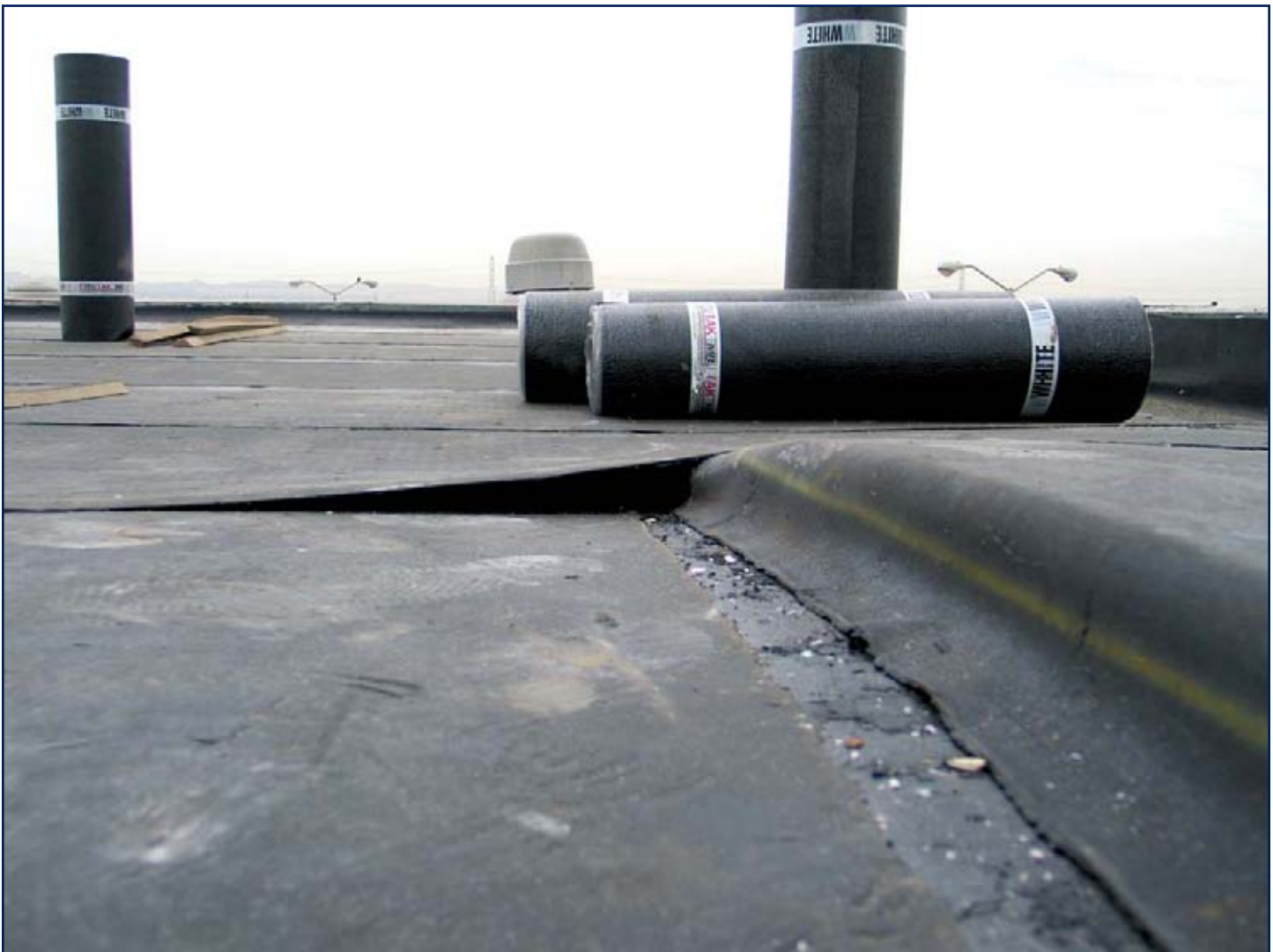
A side view showing the profile of a lifted area prior to roof cuts for visual observation.
