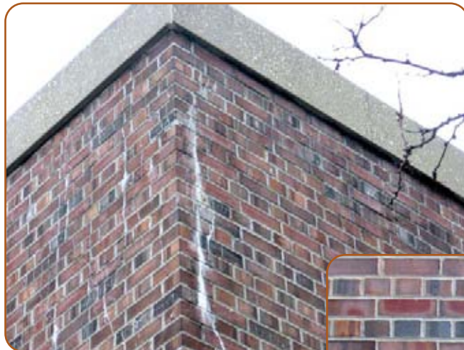
Stained, cracked masonry units.
