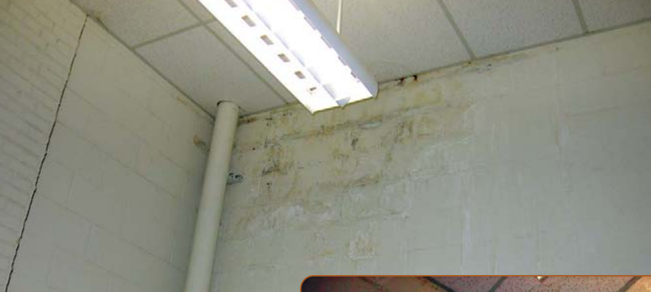
Left: Interior wall and ceiling damage.
