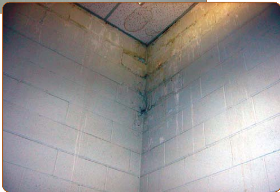
Below: Interior damage.
