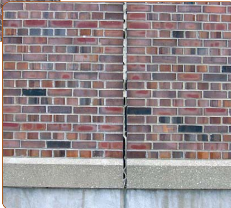
Separated expansion joint.
