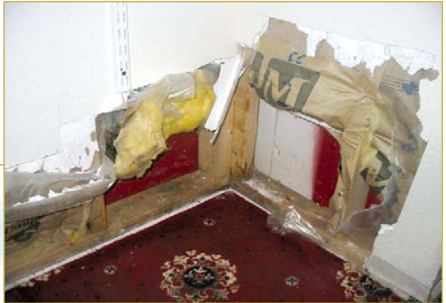
Right: Photo 1 – Damage to interior finishes at basement floor line.
