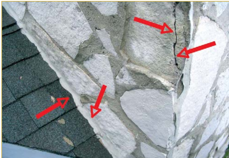
Photo 4 – Removal of loose stone cladding revealed openings in mortar bed. The shingle covering the interface with the stone cladding is sealed with caulking, restricting the harmless discharge of water from the above-roofline features.
