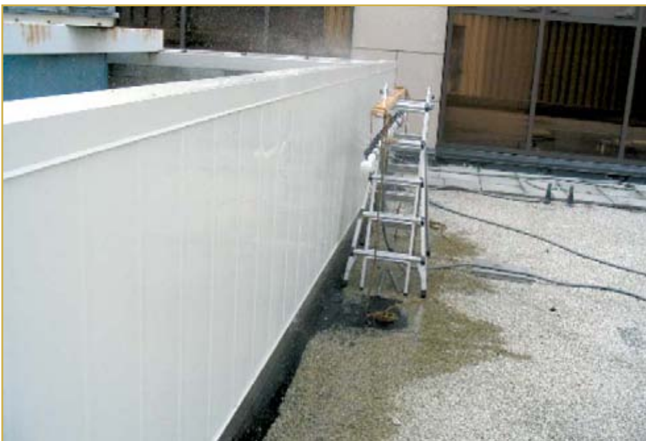
Photo 7 – Water test of the flat lock seam metal wall panel using a spray bar.
