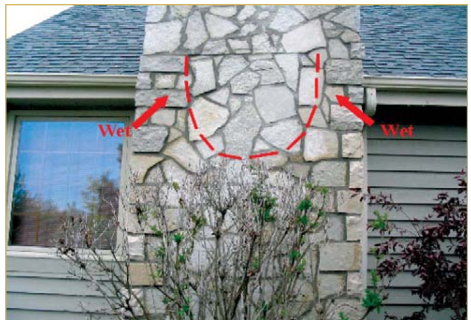
Photo 3 – The "U"-shaped pattern established as the wet stone cladding began to dry.
