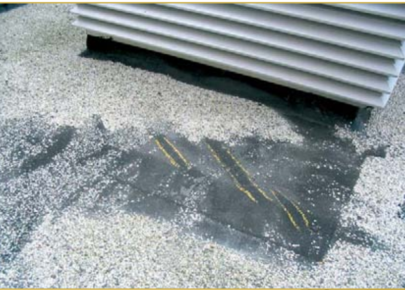
Photo 9 – Evidence of roof system movement in exposed membrane plies.
