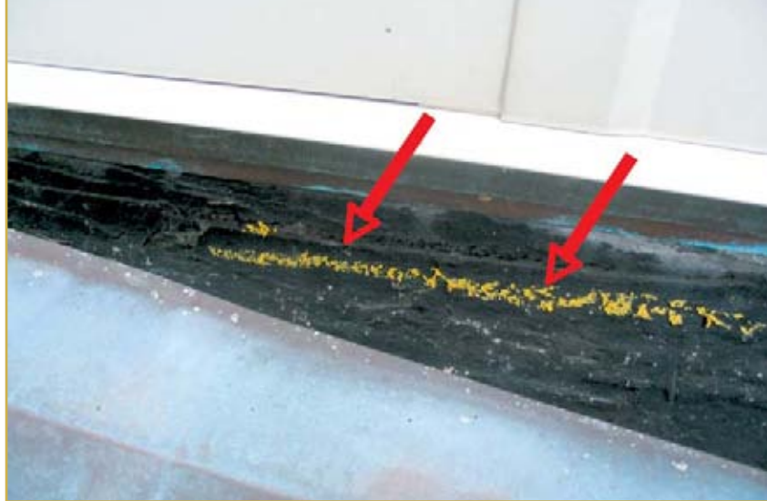
Photo 8 – Flashing termination accepting of water that moved throughout the joinery of the flat lock seam metal panel wall.
