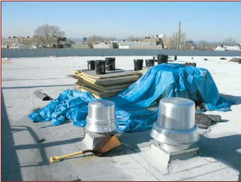
Figure 3. Improperly stored materials should not be used in the construction of a built-up roof.
