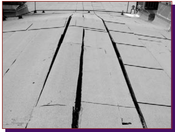
Figure 1. Cap sheet installed on steeper slope with the wrong type of asphalt.
