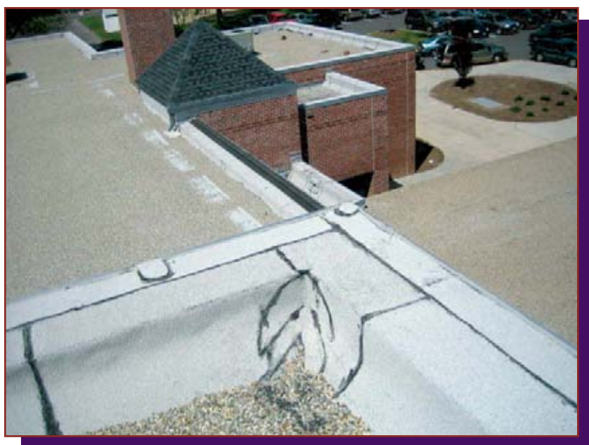
Figure 5. Flashing details are critical to the long-term performance of any roofing system.
