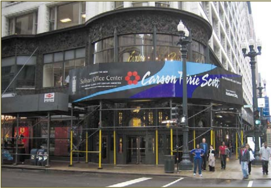
Scaffolding allows building operations to continue while work takes place above. Photo by Knickerbocker Roofing.
