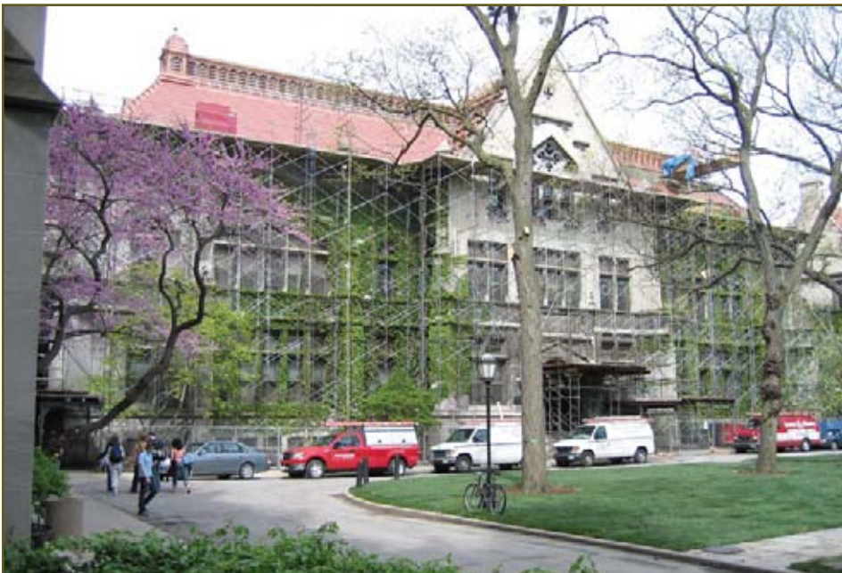
Scaffolding secures building perimeter, allowing safe egress. Photo by GILCO.
