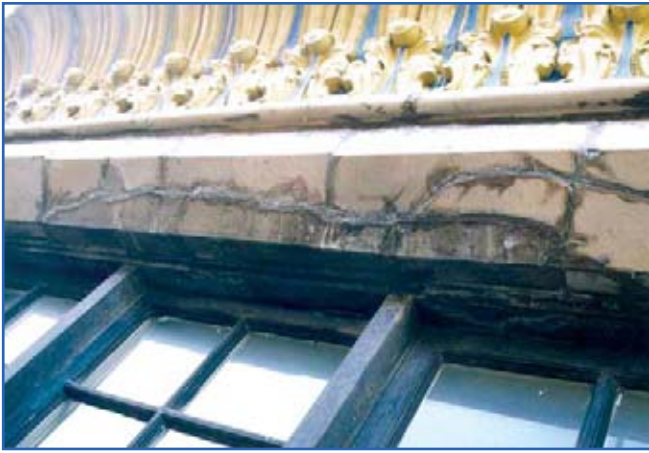
Figure 1 – Cracked masonry over a window opening is a typical condition façade inspectors should identify and classify. Knowledge of the exterior wall type is required in order to classify the condition.
