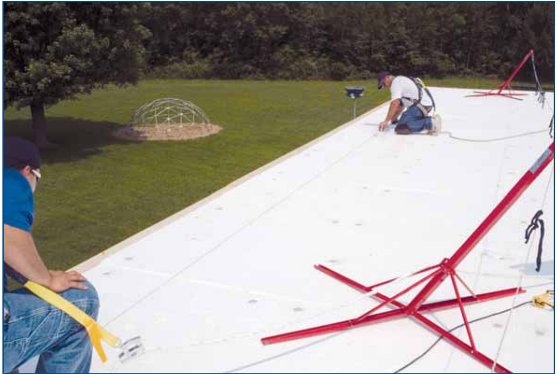
Photo 5 – Custom, pre-fabricated, single-ply roofing systems are precisely measured in advance to fit each roofing job. This reduces material waste, labor requirements and installation time, and minimizes the risk of human error by performing most of the seaming in the factory under controlled conditions. (Photo courtesy of Duro-Last Roofing, Inc.)
