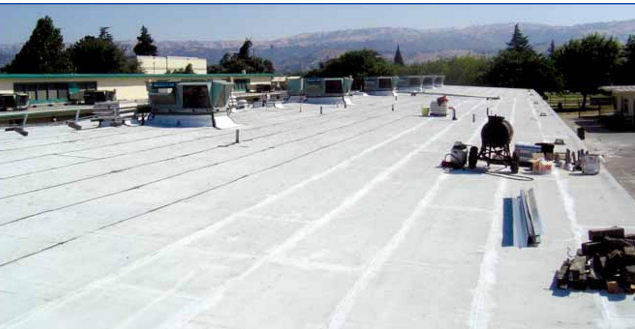
Photo 4 – Factory-coated cap sheet with field-applied touch-ups in progress. Note asphalt bleed-out at laps in left side of photo.
