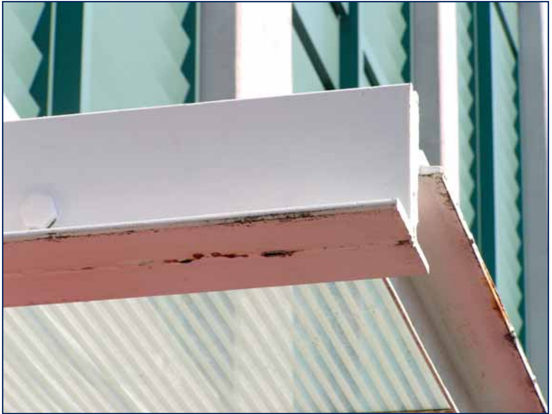
Figure 6 – Shop primer failure.
