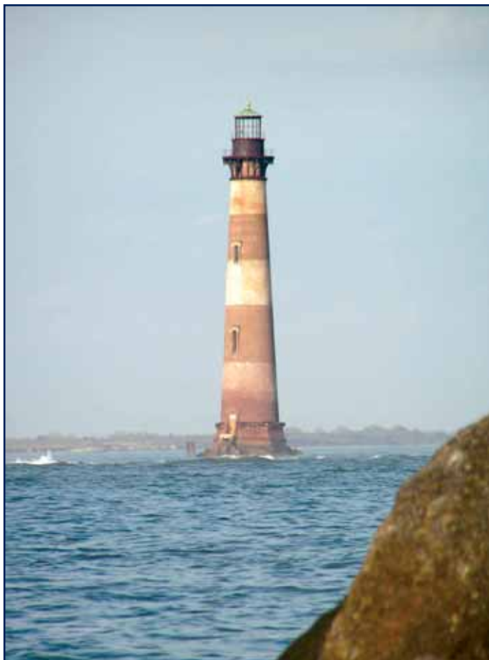
Figure 5 – Lighthouse with discolored paint.
