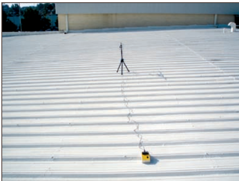
Photo 1 – Metal R-panel in North Carolina, three years old, acrylic coating.
