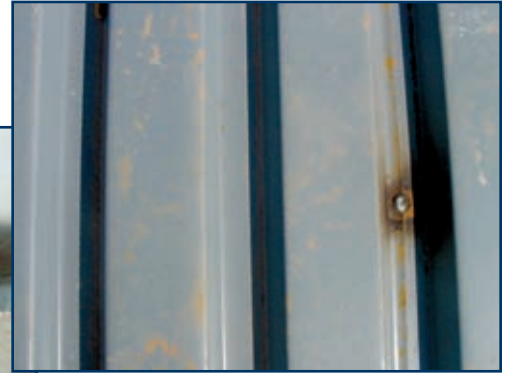
Photo 4 – Broken weld at toe of upper piece of deck (piece on left).
