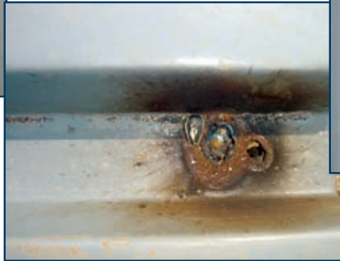
Photo 3 – Really poor-quality weld with blow-through on right side; second attempt was successful, though it is not painted yet.
