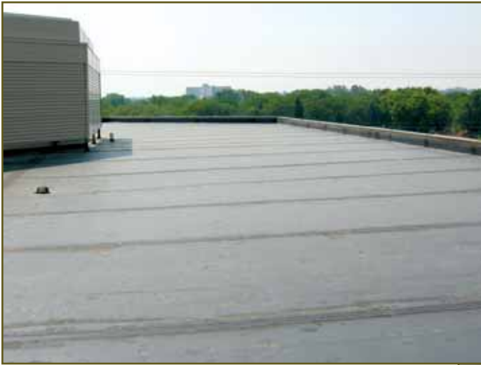
Photo 4 (left) – Note how the EPDM membrane at this drain drops into and above the clamping ring. Small details such as this communicate clearly to the owner and contractor that the designer cares about quality workmanship. (Photo by Tom Hutchinson.)
