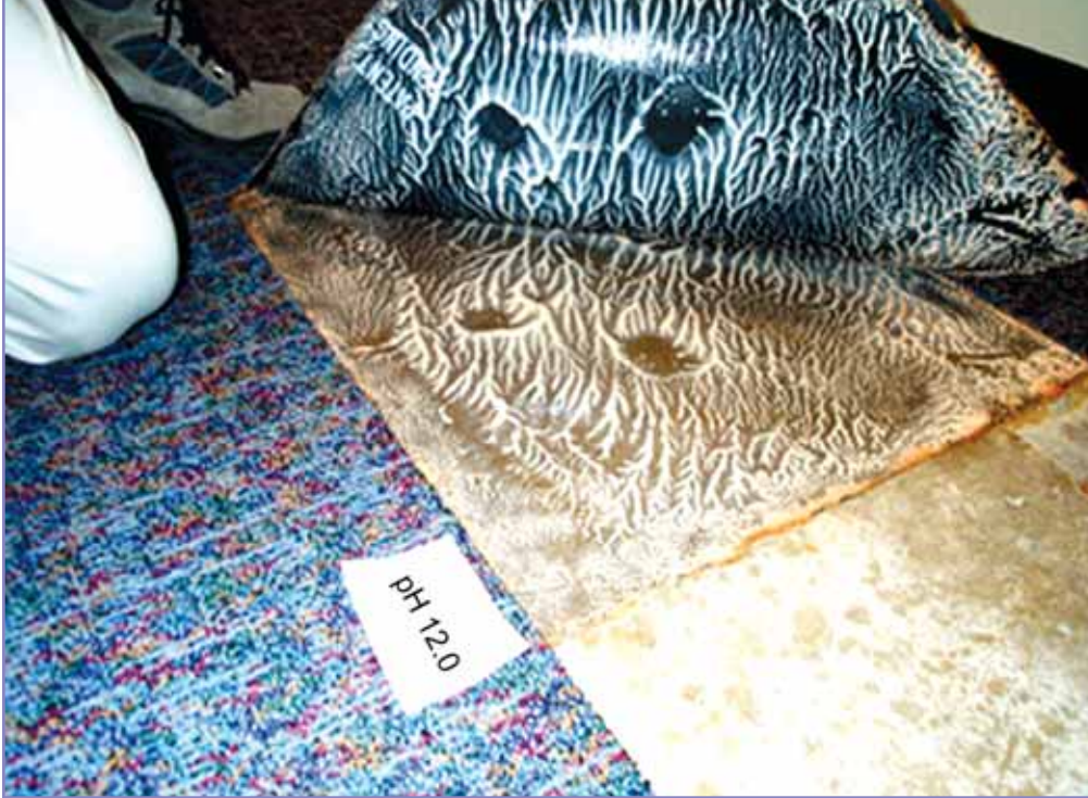
High pH condition below carpet tile
