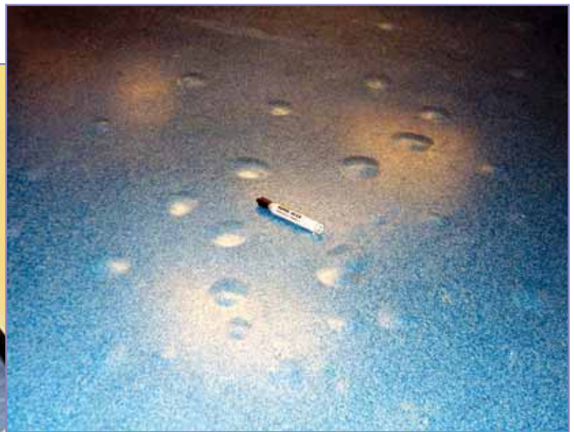
Blistered epoxy floor
