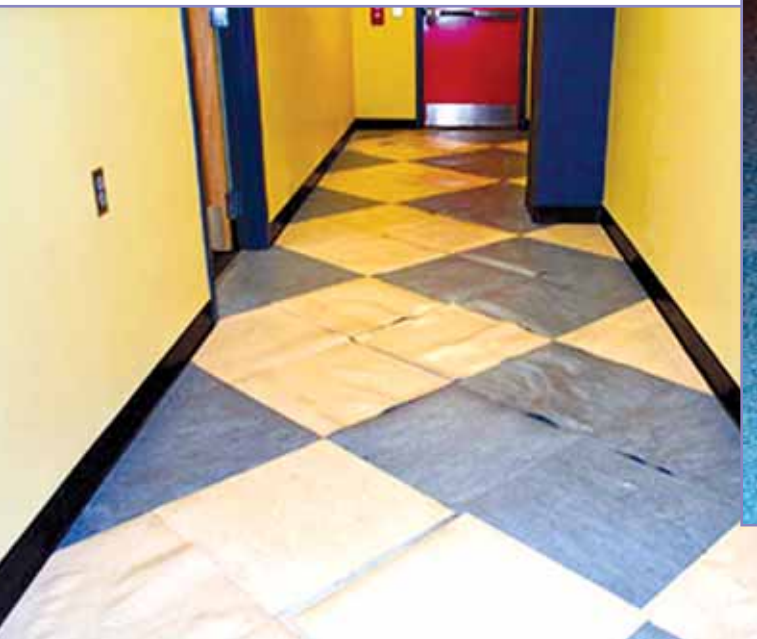
Moisture-related flooring distress
