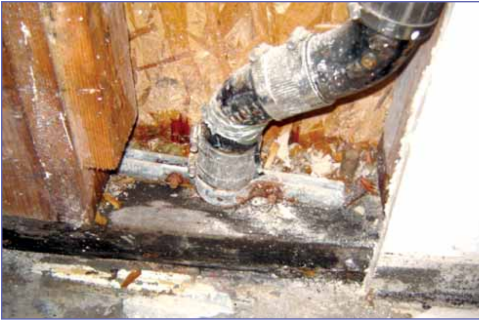
Photo 2 – Hidden leakage at drain piping connection eventually resulted in vapor condensation at a bedroom window at the opposite end of the apartment.
