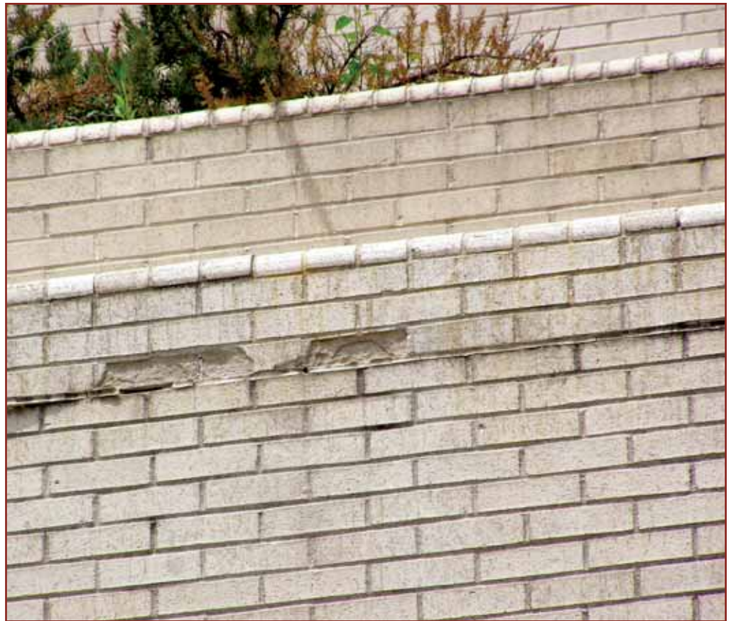
Exterior signs of brick spalling
