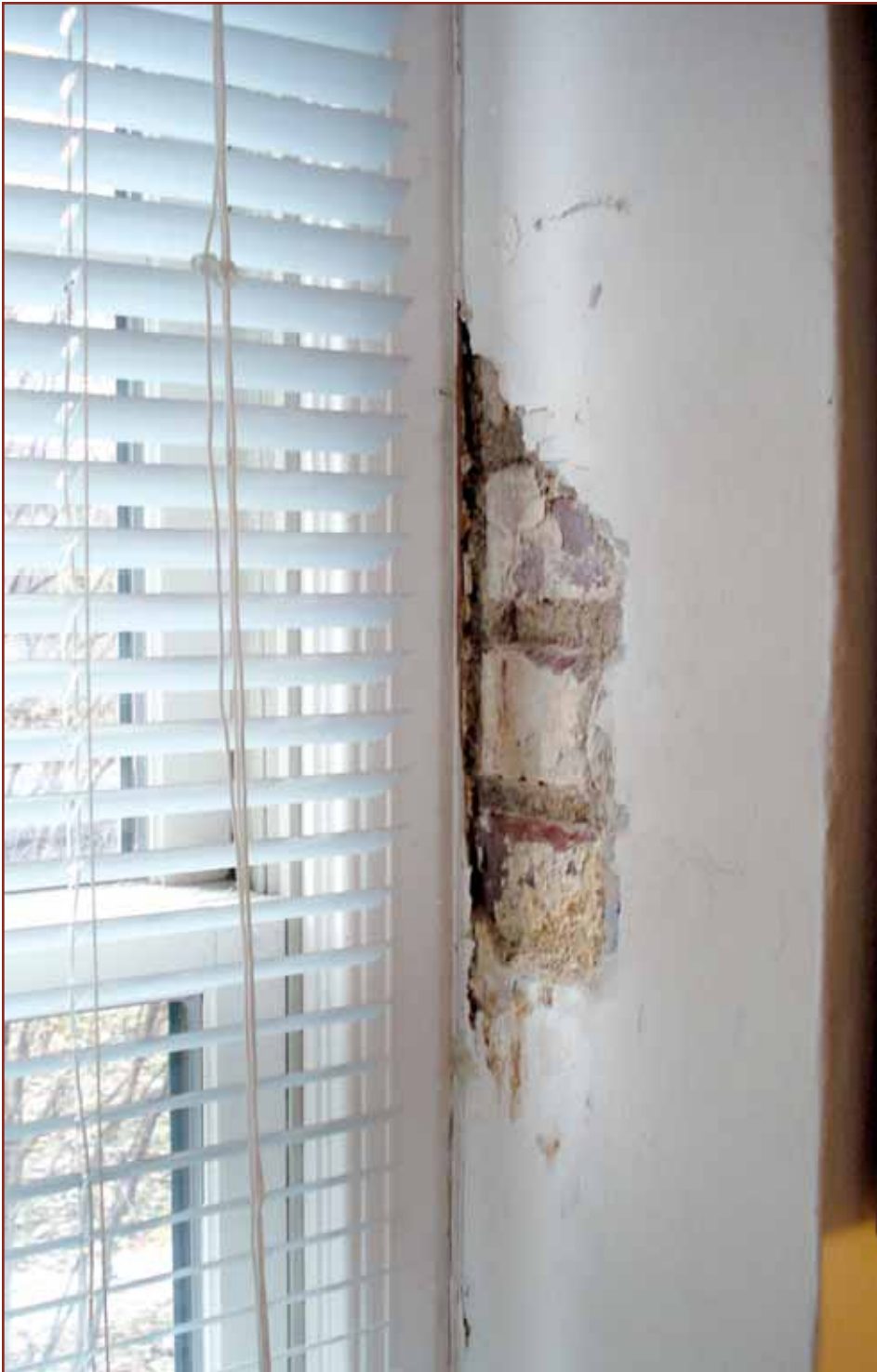
Interior damage at the jamb of a window
