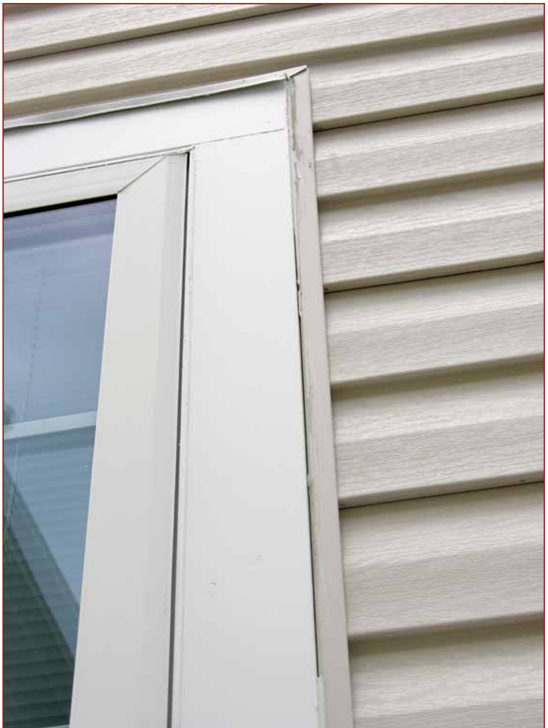
Sealant applied incorrectly at the window frame to trim and from trim to J bead
