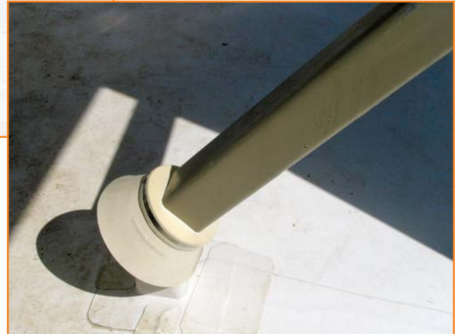
Photo 6 – Close-up of 6-inch, angled storm collar.
