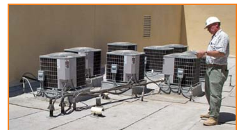
Photo 4 – Split central air-conditioning units on the Trammell Crow roof.
