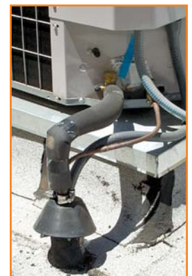
Photo 3 – Closeup of a line set at the Trammell Crow project.
