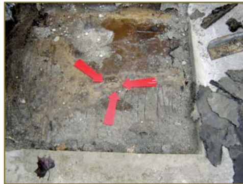
Photo 3 – Typical breach in the overly thin, nonreinforced, fluid-applied waterproofing membrane.
