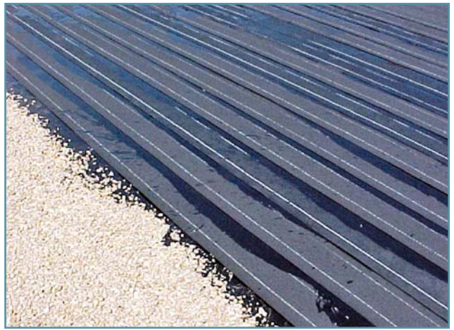
The layering technique for applying the reinforcing plies, topped with aggregate embedded in a flood coat of coal tar roofing pitch, maximizes the life span of this roofing system.
