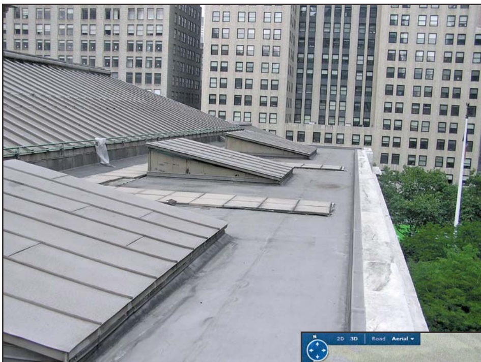
Photo 7 – Photo taken from the roof above the 5th Avenue entrance to the library.
