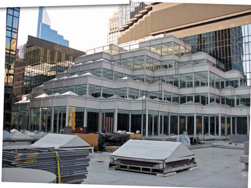
Daily work areas were set up to provide a work platform and a safe work zone and to protect the existing structure.
