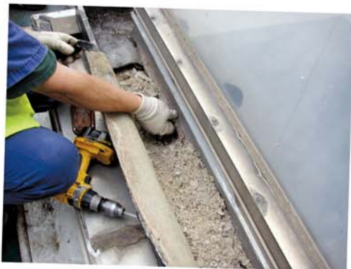
Past moisture intrusion damaged the lightweight concrete deck.
