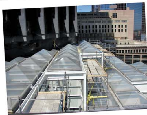
Scaffolding was erected to provide a safe working surface at the leading edge.
