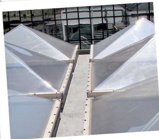
10-inch spaces between the skylights limited the work space and made material delivery challenging.
