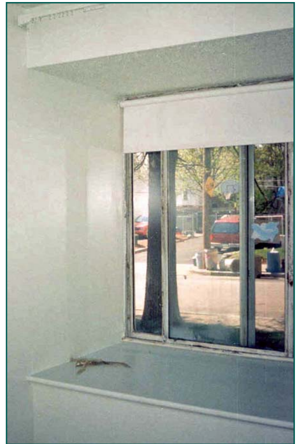
Photo 1 – Bay window with restricted access due to deep interior-sill dimension.
