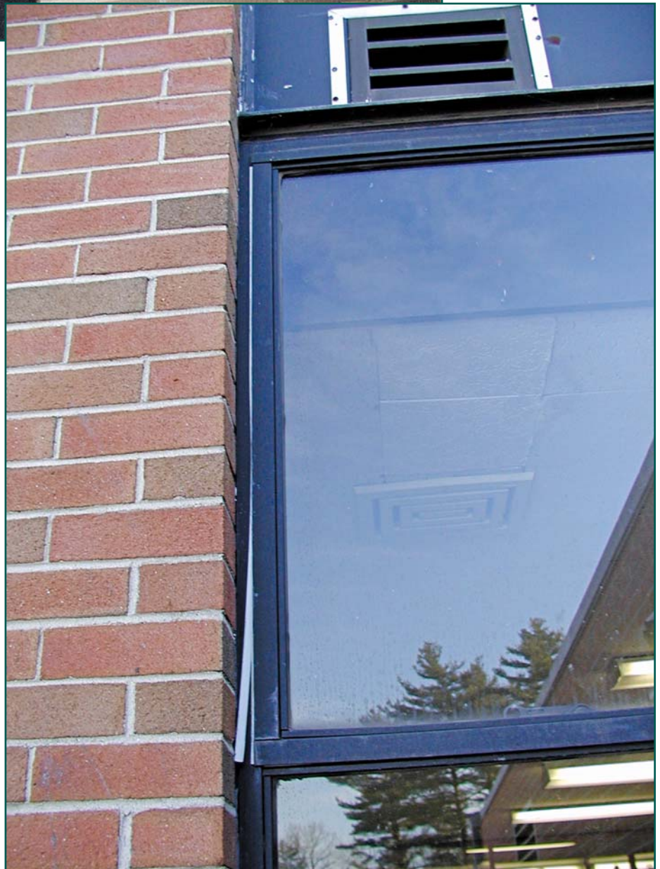
Photo 3 – Air leaks through sash/frame connections.
