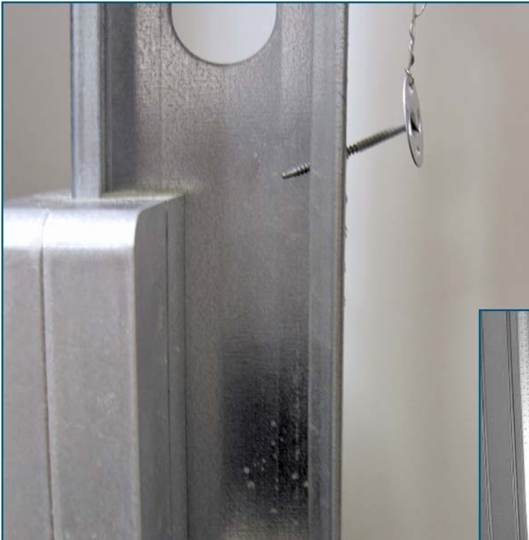
Photo 1 – Fasteners in deflection.
