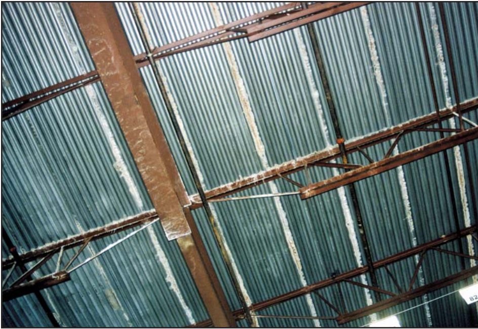
Figure 3 — Often mistaken for a “metal deck,” LWIC is most commonly carried on a metal “formboard.” Modern iterations have slots at the bottom of the flutes/ribs to liberate construction water and induce continued drying. This image depicts an older version that predates slotted decks. The material emerging at formboard edges dates to the day it was installed and should not be confused with active leakage.
