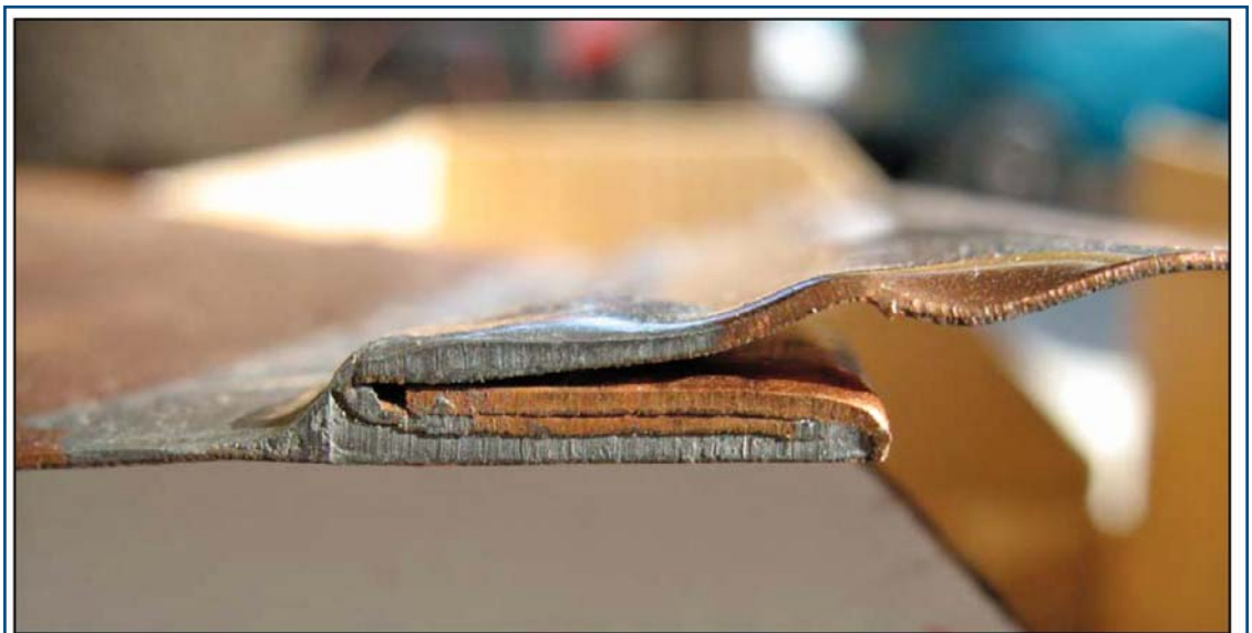
Figure 2.9: A poorly soldered sample seam. There is little solder within this locked and soldered seam. The solder is primarily surface applied. Seams such as this will fail within months after installation on a roof.
