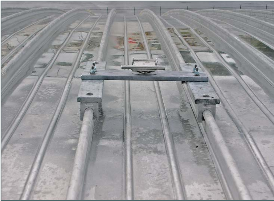
Photo 3 – Example of anchorage points with horizontal lifeline installed on a standing-seam metal roof at Northwest Florida Beaches International Airport. Illustrates plan point of view similar to configuration depicted in Figure 2. System is designed for fall-arrest requirements only. Photograph courtesy of Pro-Bel.
