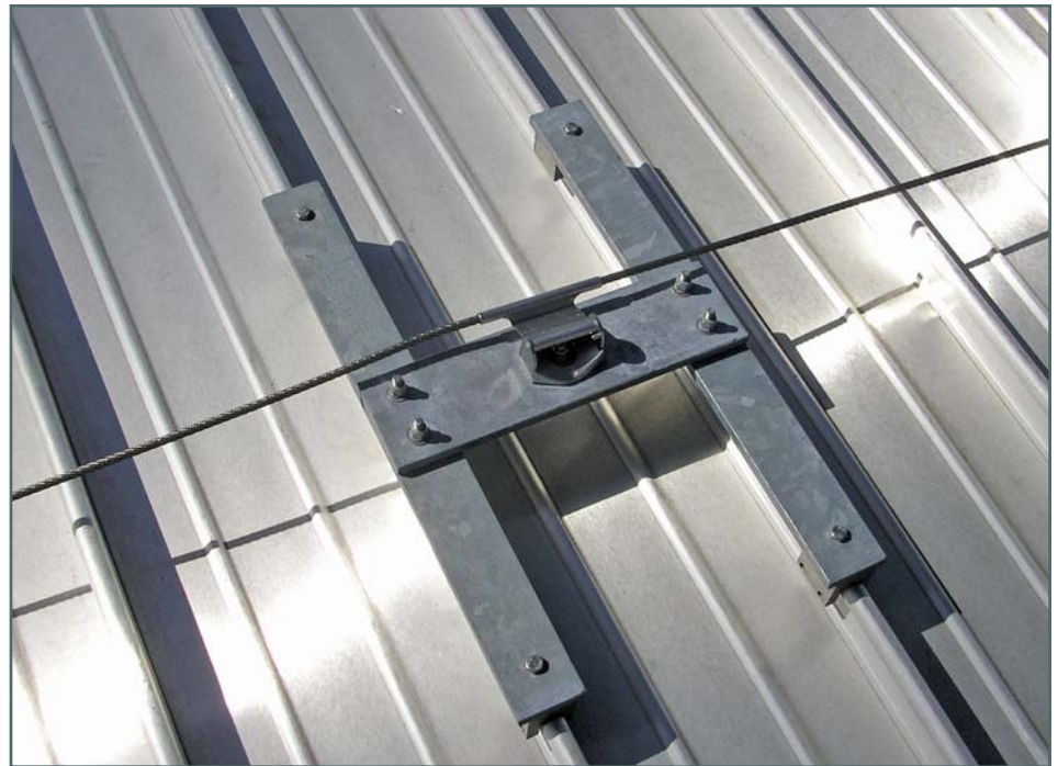
Photo 2 – Example of anchorage points installed on a standing-seam metal roof at Northwest Florida Beaches International Airport (horizontal lifeline not yet installed). Illustrates cross section point of view similar to configuration depicted in Figure 2. System is designed for fall-arrest requirements only. Photograph courtesy of Pro-Bel.
