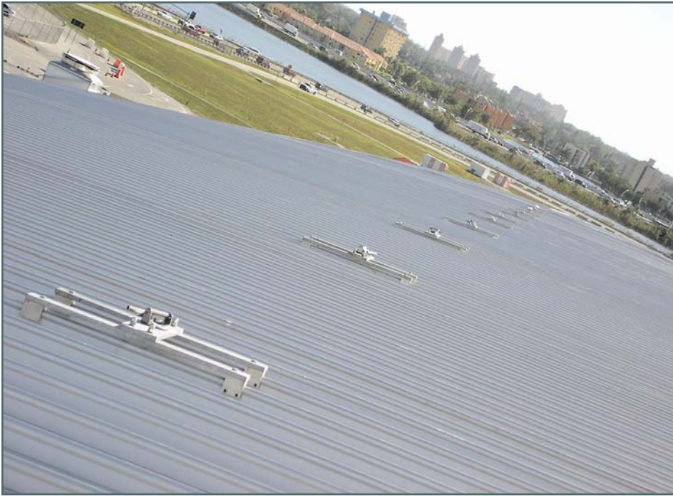
Photo 1 – Example of anchorage points installed on a standing-seam metal roof at Northwest Florida Beaches International Airport (horizontal lifeline not yet installed). System is designed for fall-arrest requirements only. Photograph courtesy of Pro-Bel.
