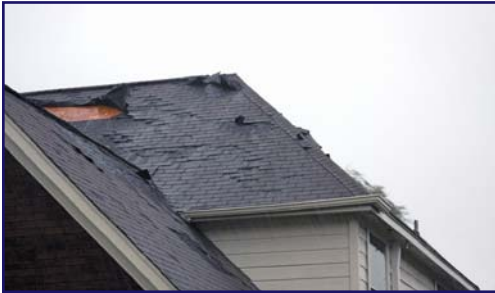
B. A large number of shingles blown off.
