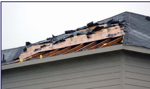
C. Heavy damage as a result of shingle and sheathing loss.
