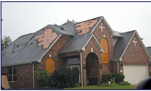
A. Widespread damage to roof shingles.
