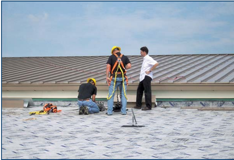
Figure 4 — Metal panels are being installed over PS200HT self-adhering underlayment, which provides a smooth surface and resistance to high temperatures.
