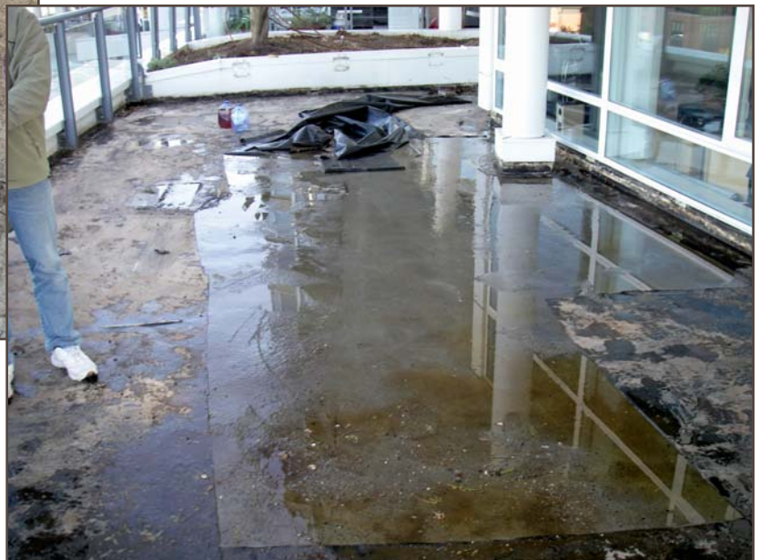
Figure 4 – Water beneath blistered membrane over entire deck.
